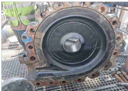
Bolt Engineering and Distributors (B.E.D.) is synonymous with safety and quality.
